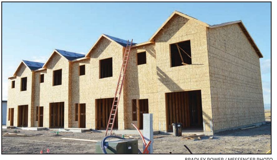
The first of five flourplexes going up on 700 North 100 East, one of more than 80 family units under construction or recently completed in Ephraim. An apartment development that could have up to 80 units has been approved on the same block.
